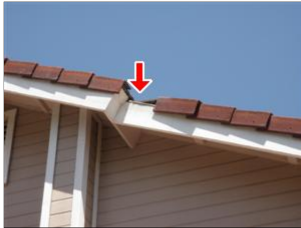
9.0 Picture 1 Missing tile
