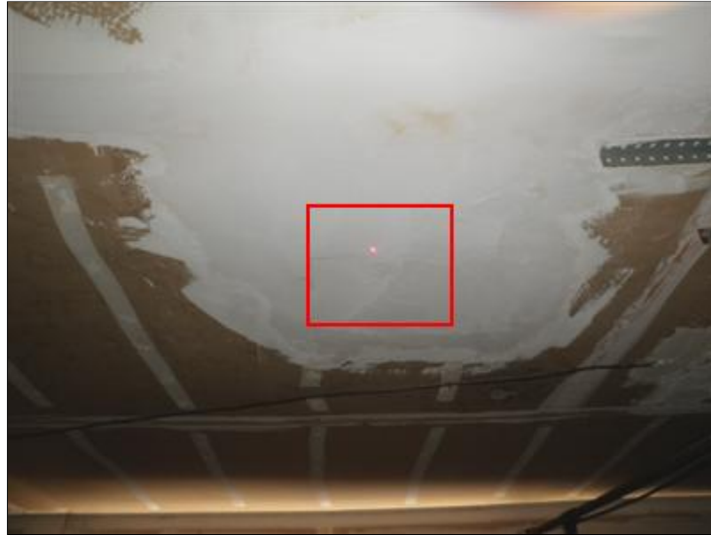
6.1 Picture 5 Leak below master tub/shower in Garage
